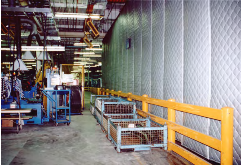
Typical 'ABA; style curtain array separating large work areas.
